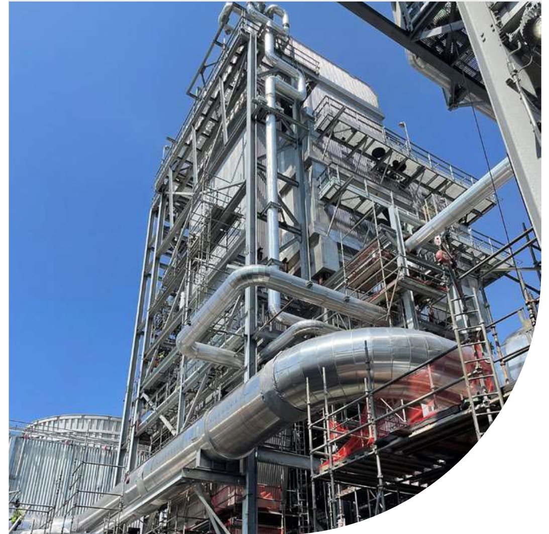
Orion's plant in Ivanhoe, Louisiana.
